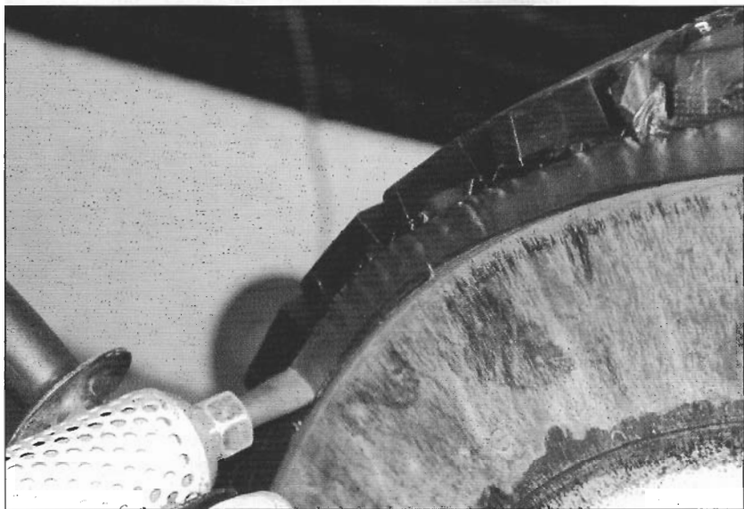
Photo VI - In some cases, the shoulder design is filled with a hand-held extruder gun.
